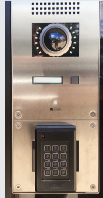
An IACS-installed access system, featuring a Farpointe Data Reader & Keypad
