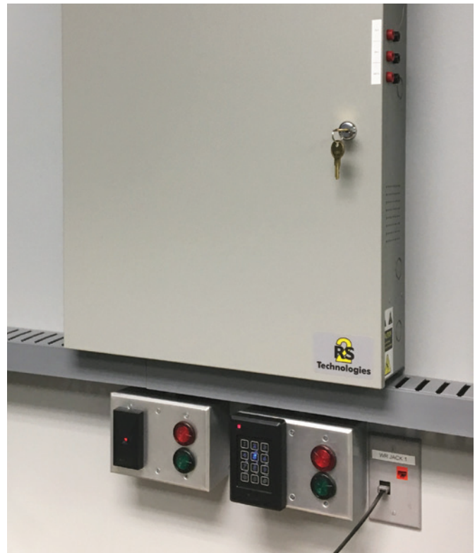
IACS's tech team thoroughly tests each component of their integrated systems. Above, Farpointe Data's P-300 Proximity Reader and P-640 Proximity Reader & Keypad are tested with an RS2 access control panel.
